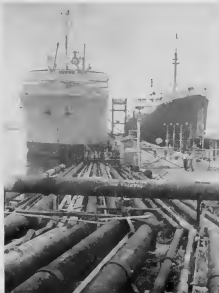
The pipelines leading down to the pier are clearly marked and painted. (The Kosmos III fueled on two 16" lines.) Another difficult factor in loading whalers is their top-heavy construction, which means that the loading of oil and discharging of ballast must be timed to keep the ship on an even trim.
